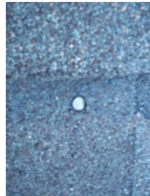
Exposed nail below dryer vent.
