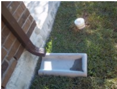
Splashguards turned around wrong, so they will hold water.
