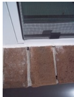
Gap in brick sill mortar over porch
