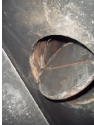
Damper will not close due to metal of flue.
