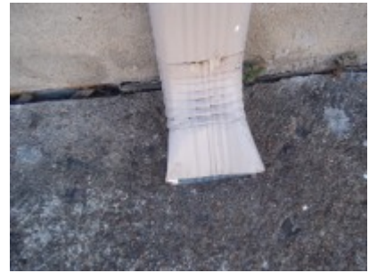
Damaged downspout rear.
